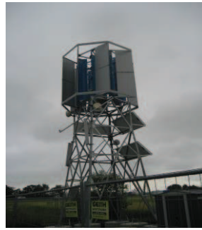
Fig. 2. Installation of a 4kW Turbina VAWT free-standing for example in industrial park areas.
